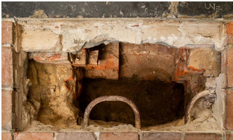
Figure 1. Ledger stone of Anne Randall, St. Luke's Church, with heating pipes visible in the open pit next to the burial chamber.
